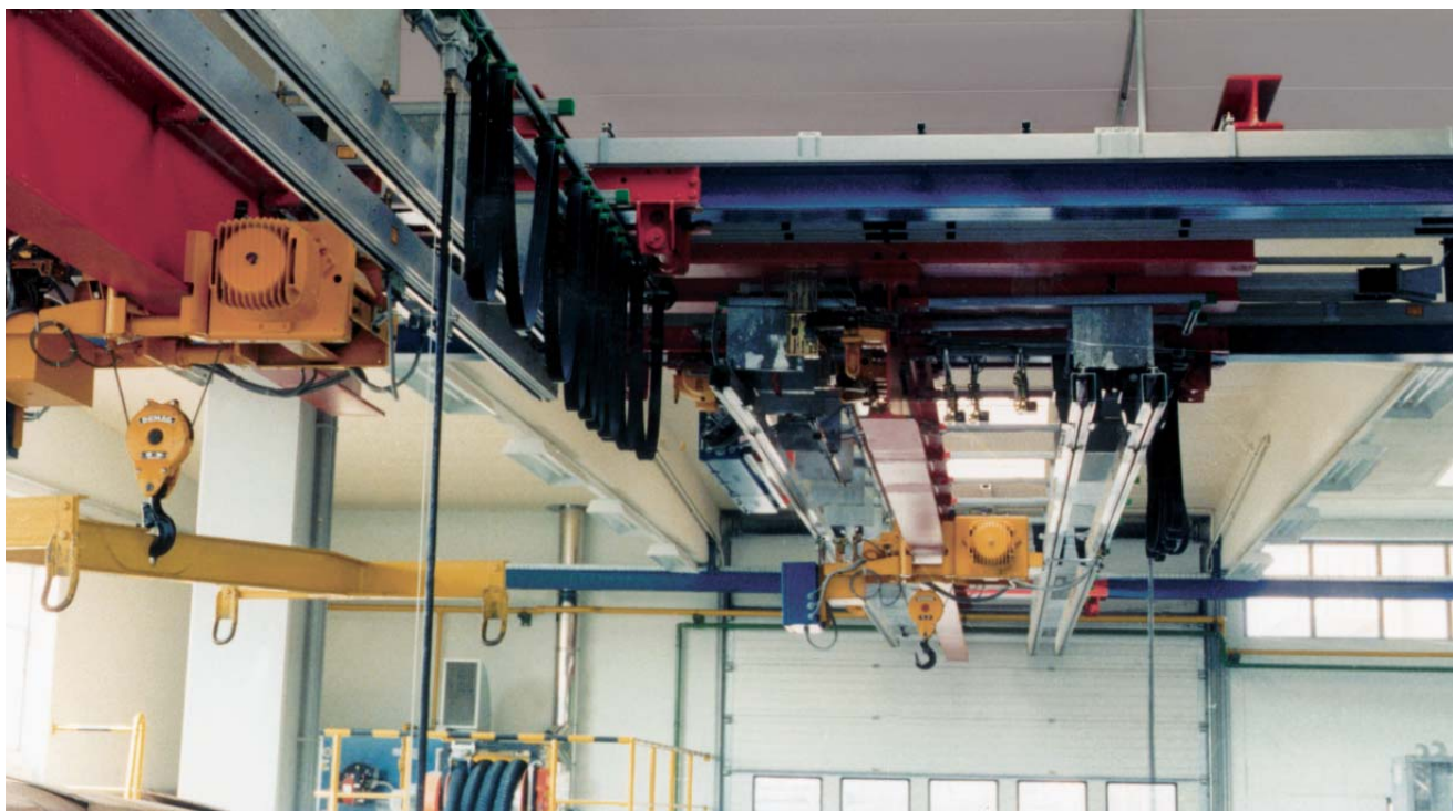
Aluminium enclosed conductor system on crane bridge.
