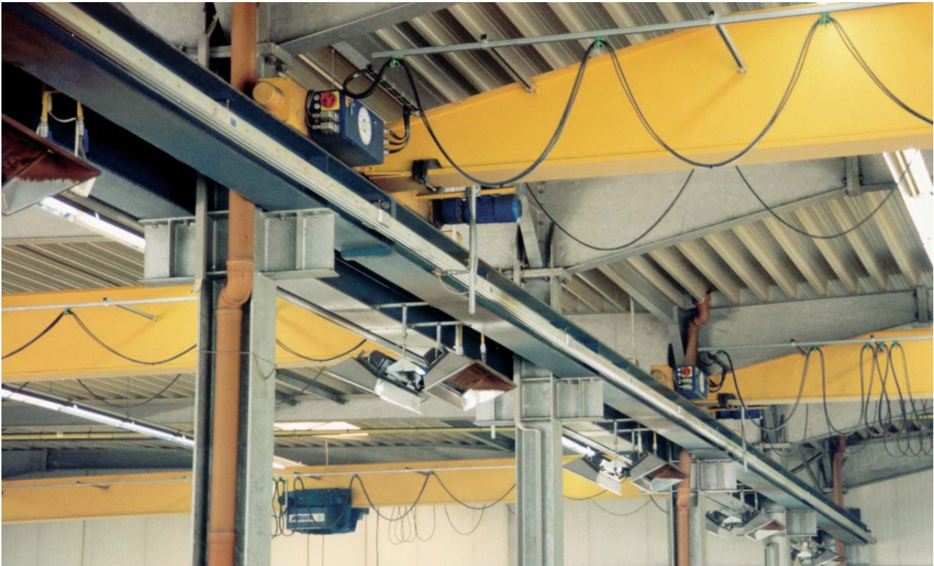
Aluminium enclosed conductor system for crane electrifications.
